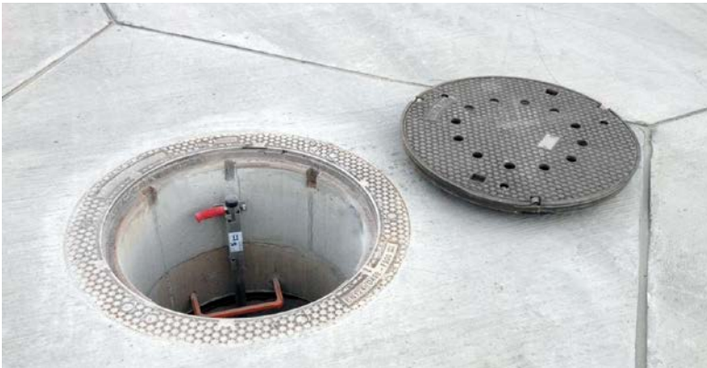
Cast-iron cover with screw-in locking lever fastenings, a load class of F 900 and a clear opening of 800 mm
