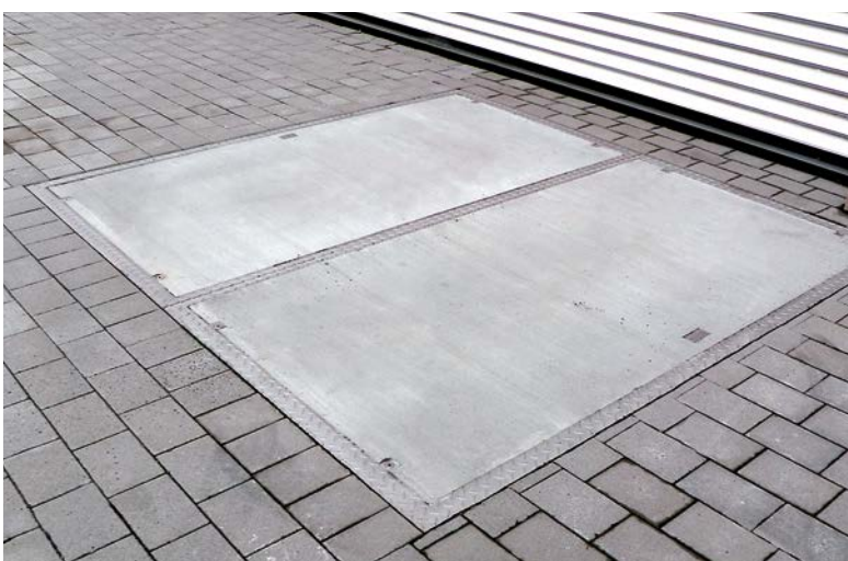
Two-piece shaft cover with concrete surface, Frankfurt
