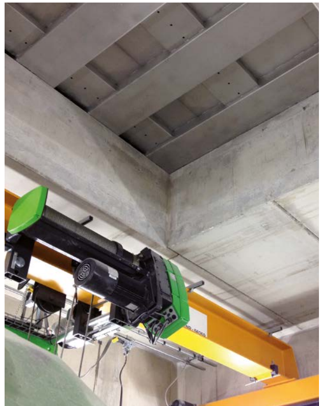
View from below of a floodproof cover on an assembly opening, power plant on the river Danube near Augsburg
