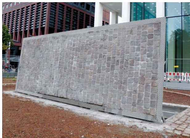
Escape hatch with paved cover, Frankfurt
