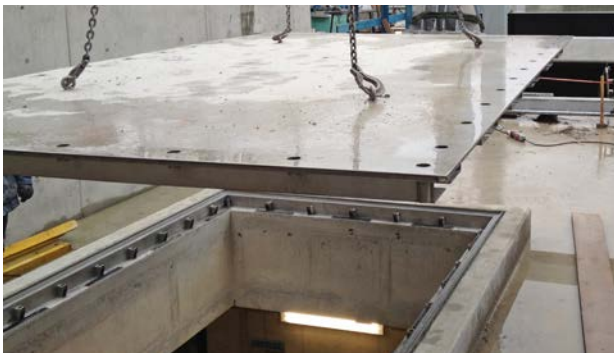
View from below of a floodproof cover on an assembly opening, power plant on the river Danube near Augsburg
