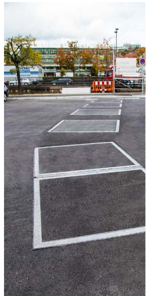
Backwater-proof covers filled with asphalt, Ansbach
