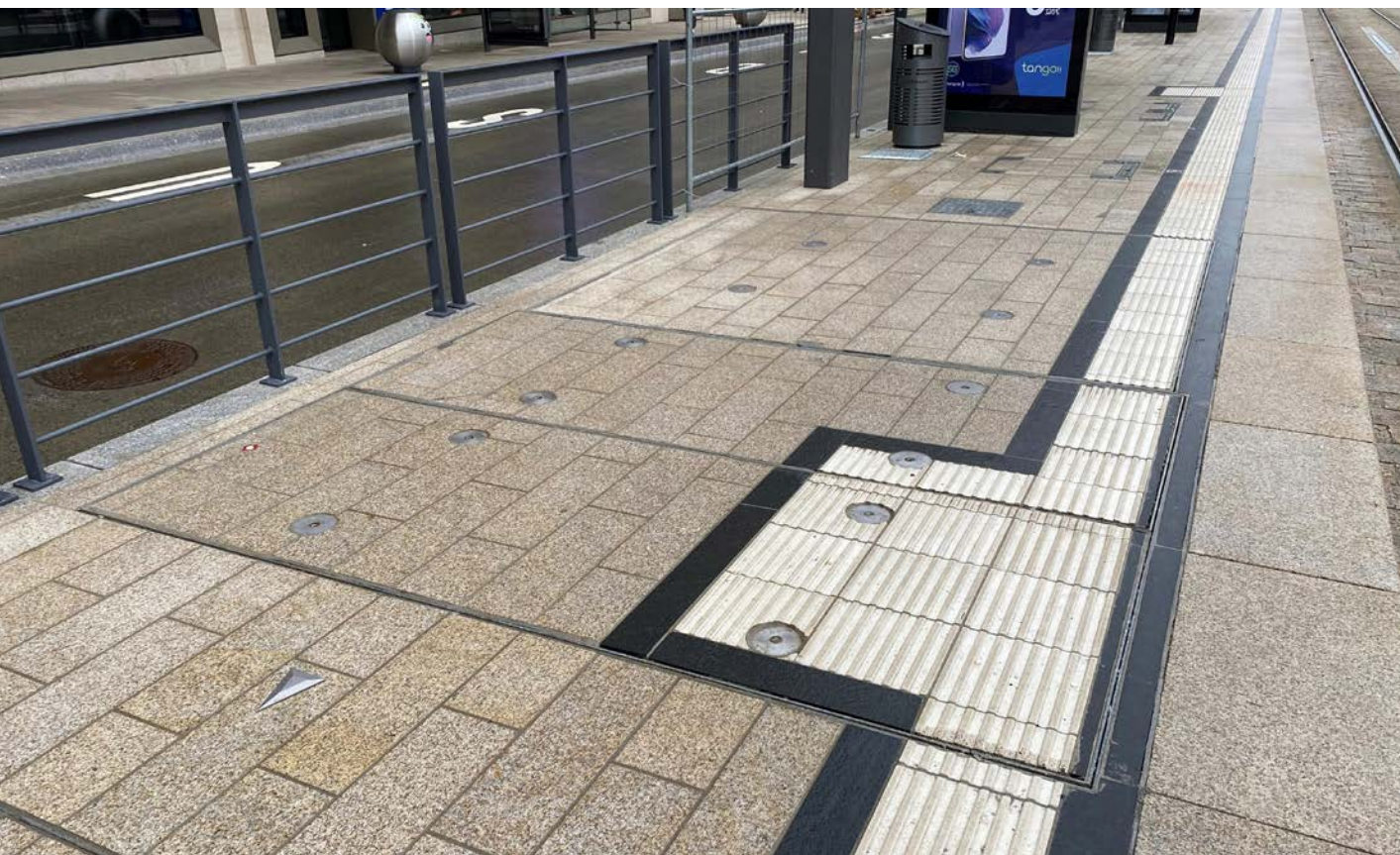
Discreet, as little metal on the surface as possible – this can be realised with pavalbe floor hatches, Luxembourg
