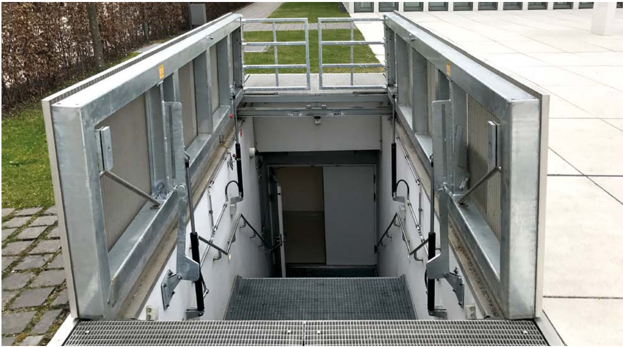
2-piece floor hatch as an emergency exit, Munich
