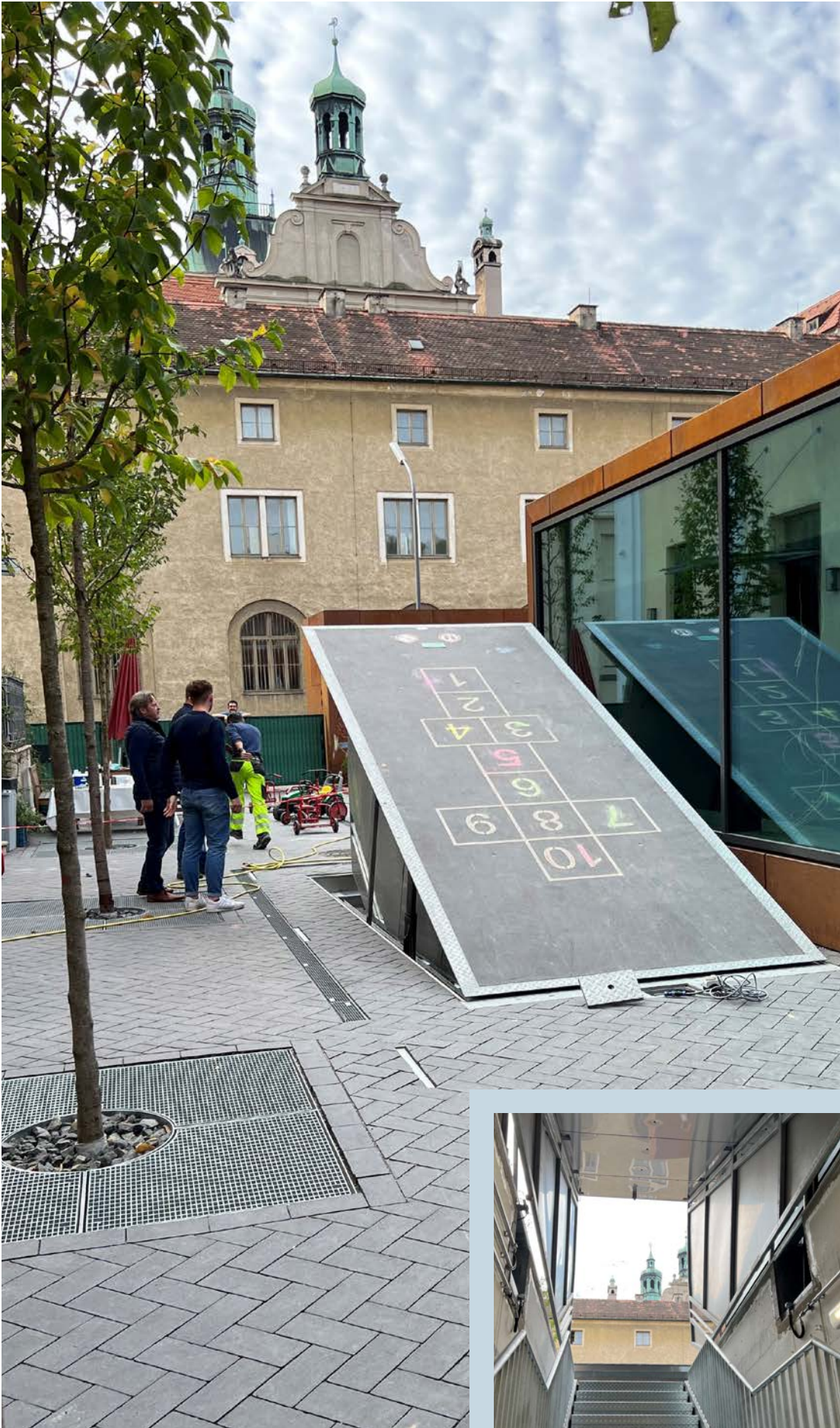
Automatic opening even in the event of a power failure thanks to hydraulic pressure accumulators with integrated emergency power supply, Munich State Archaeological Collection
